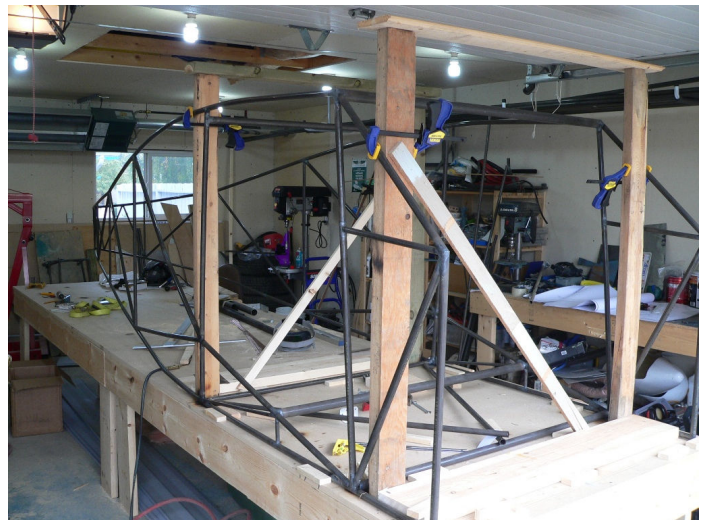
The fuselage is now standing with the first few cross members installed. At this point, the frame is ready to have a temporary seat installed so you can get a little stick time...
